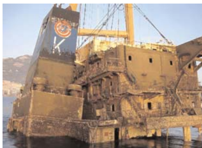
Titan reported in August the removal of the 600 tonnes accommodation block from the wreck of the bulk carrier New Flame .
