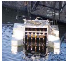
Waste Water Treatment Skimmers
